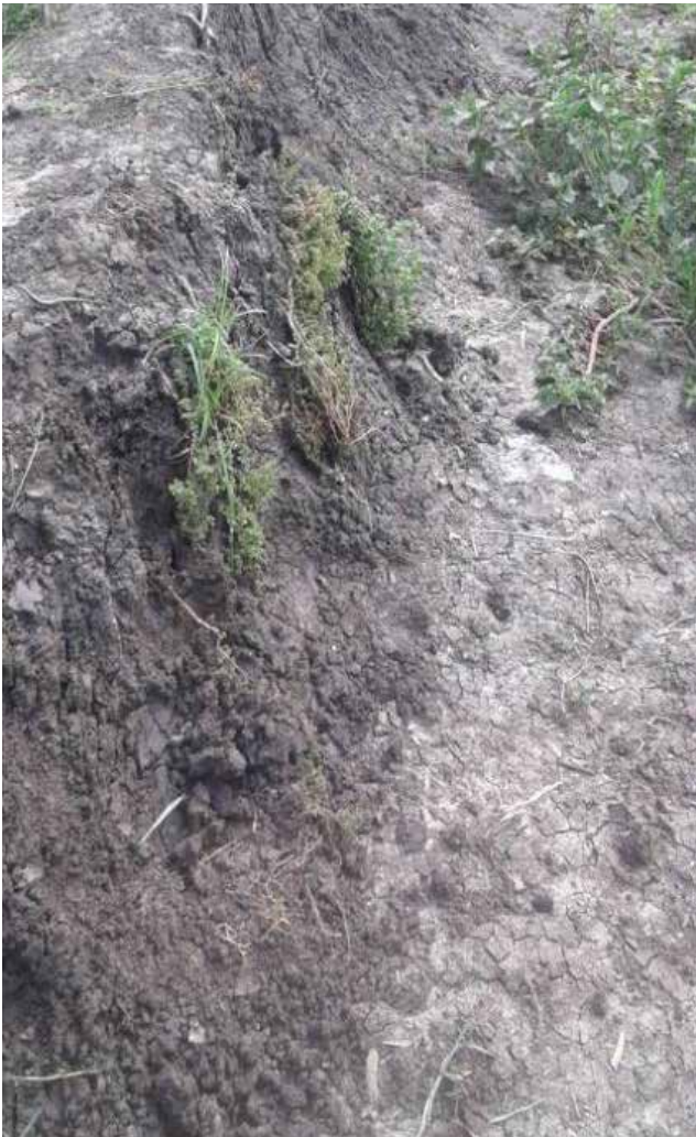
Figure 17. Degraded dyke in Jikmir, Nasir.
