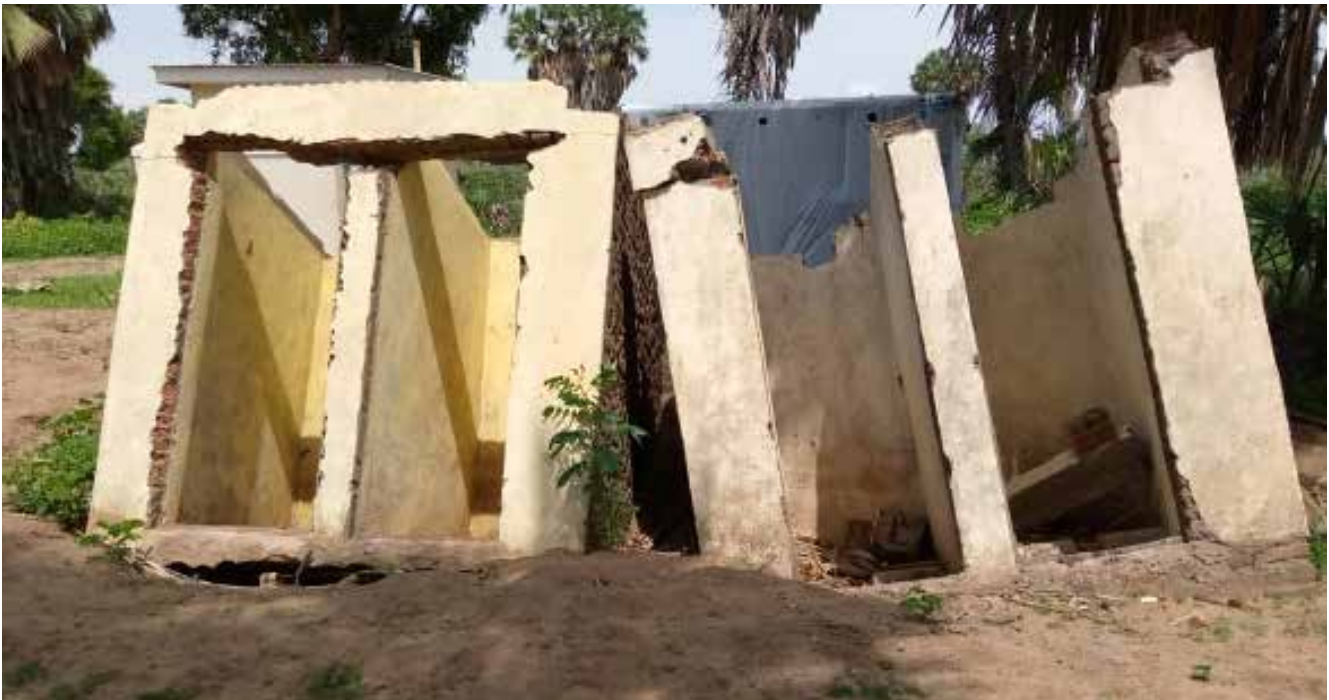
Figure 5. Damaged latrines at a local school
